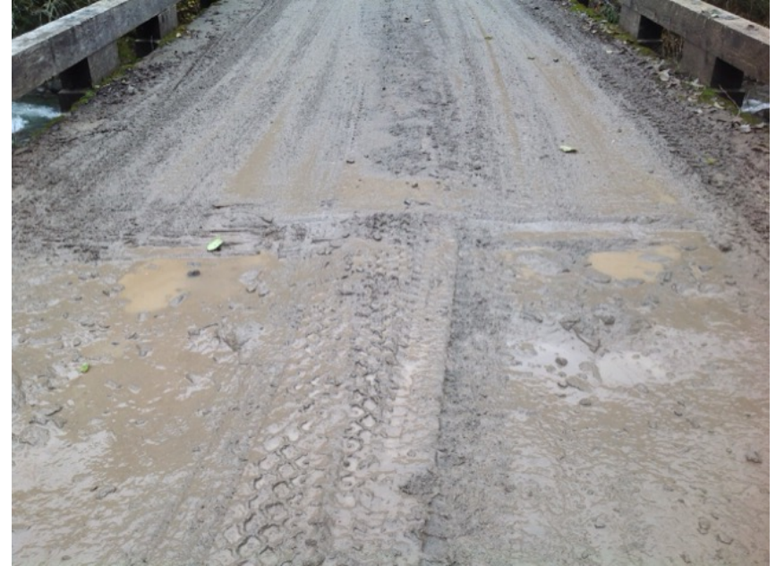
potholes at approaches
